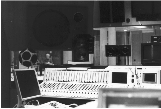
Figure 4.15: Control room of Studio 3 in the Danish Radio, Fredriksberg, Copenhagen
